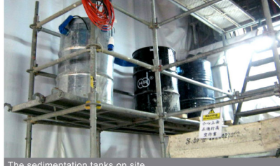
The sedimentation tanks on site
